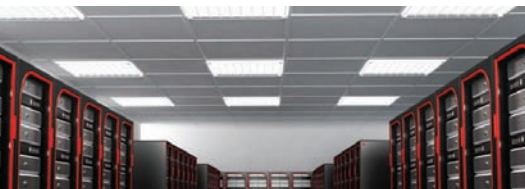
Server Room Monitoring
